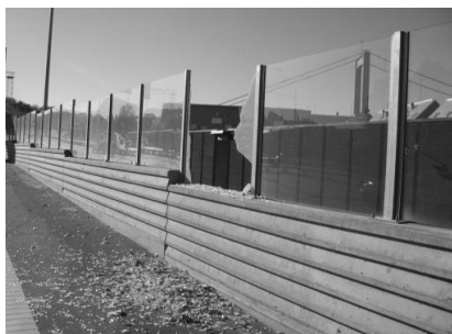
Figure 1.1 Damaged noise barrier along road E6 in the city of Gothenburg in Sweden
