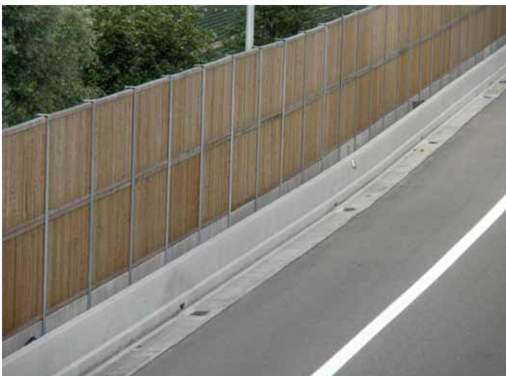
Example of a concrete step barrier installed in front of a noise barrier
