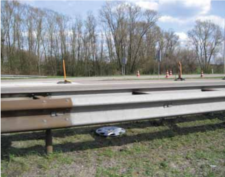
Example of corrosion of a steel guardrail
