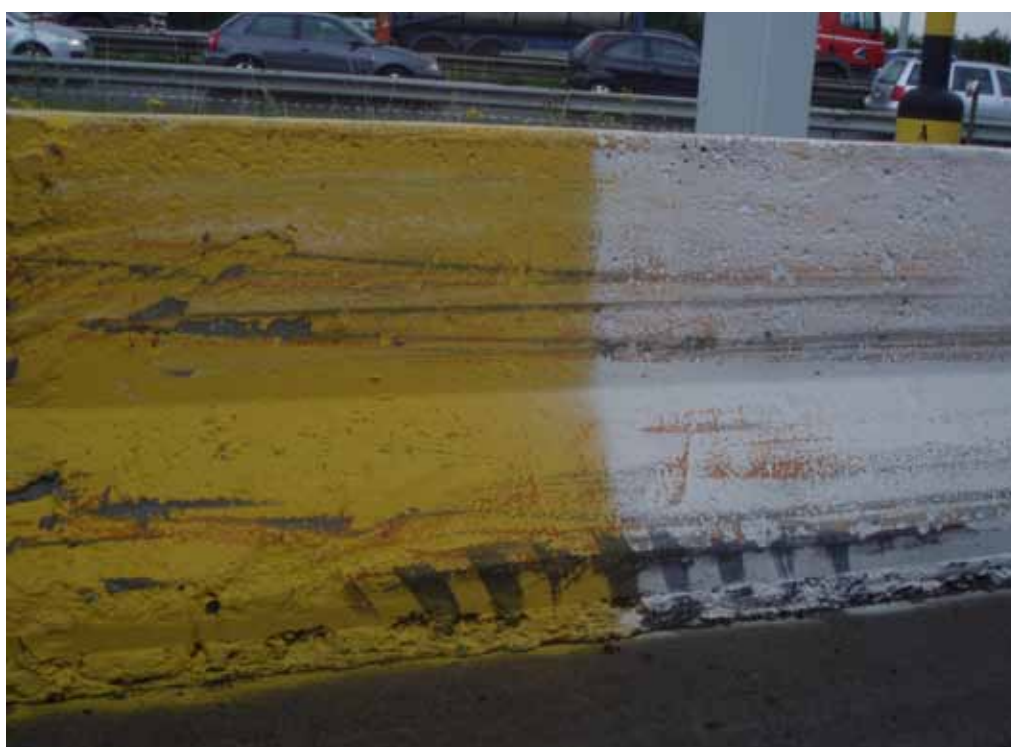
Traces of tyres on a concrete safety barrier, showing its resistance to vehicle impacts
