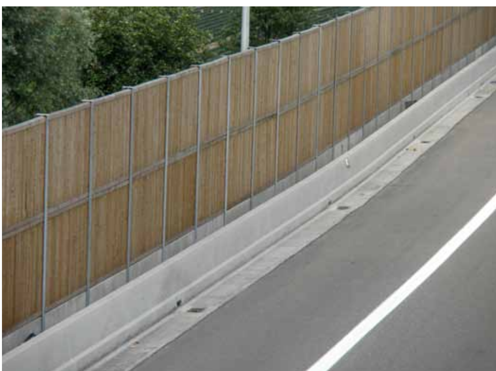
Example of a concrete step barrier installed in front of a noise barrier
