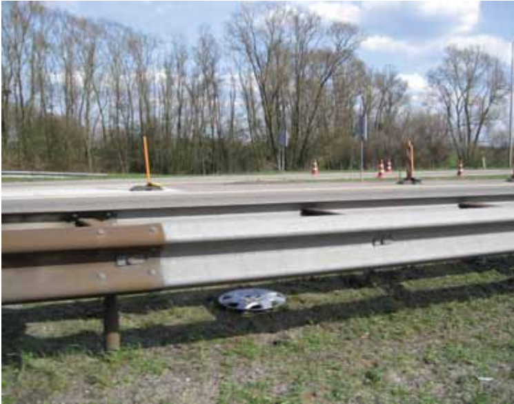
Example of corrosion of a steel guardrail
